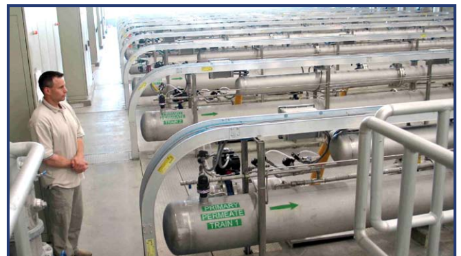
Figure 54b. Pipes within the treatment plant contain the membrane filtration units. (Photo by R. Turner)
